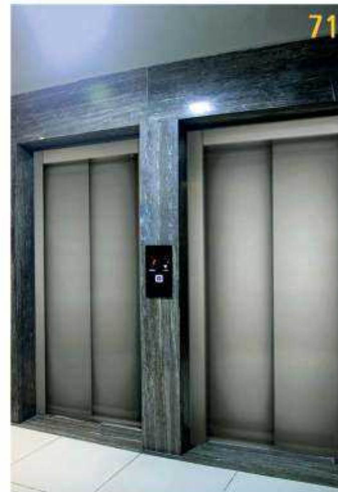
71 PROJECT NAME: AMIRIYE COMERCIAL, OFFICIAL COMPLEX CLIENT: JAHROM BETON COMPANY ELEVATOR TYPE: TRACTION YEAR OF CONSTRUCTION: 2015/ 2016 NUMBER: 2 ELEVATORS
